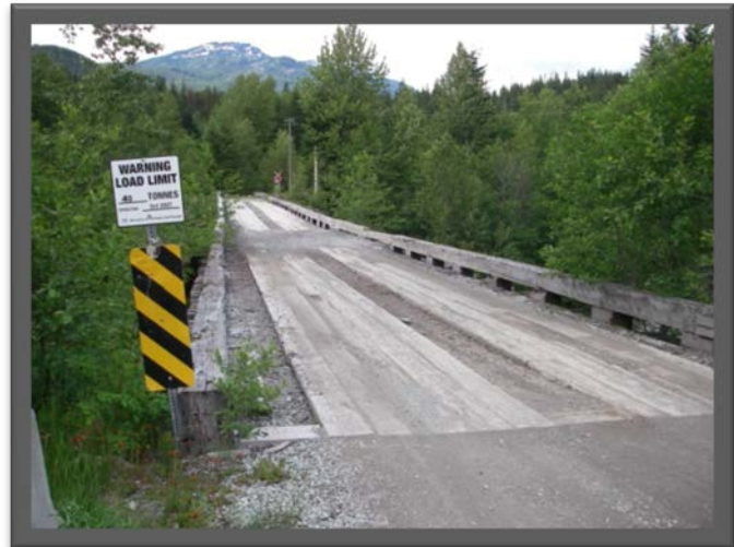
Bridge with load restrictions posted.
