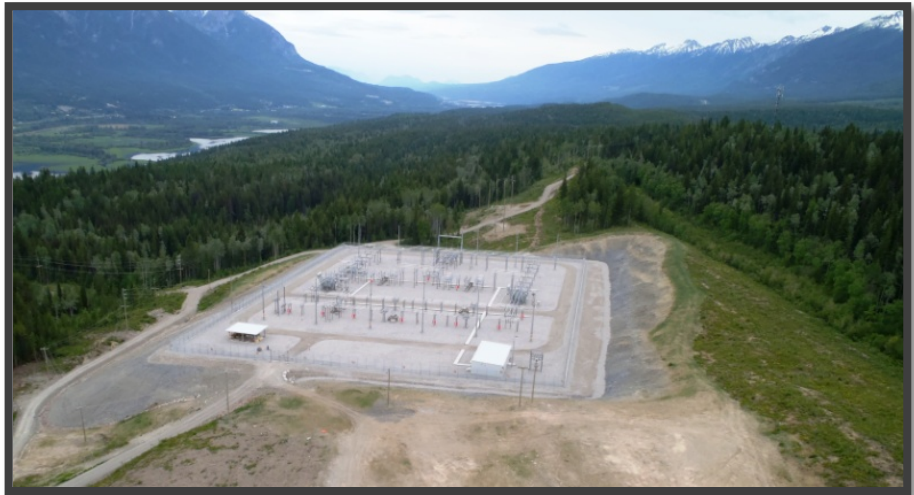
Kicking Horse substation, west of Golden, BC and the Columbia Valley transmission line extending south towards Invermere.
