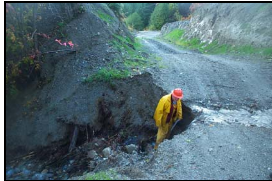
Example of a deactivated crossing where the road fill was not excavated to the original stream channel. Erodible soils were not sufficiently armoured or pulled back from the streams channel to minimize sedimentation into the streams.
