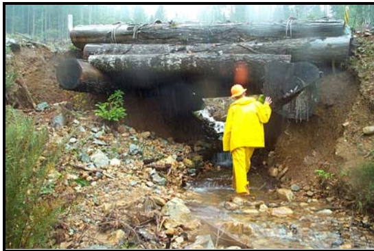
Example of a crossing structure perched on road fill and not adequately armoured, introducing sediment directly to the stream.
