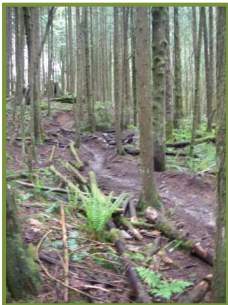
Trail with inadequate surface drainage.
