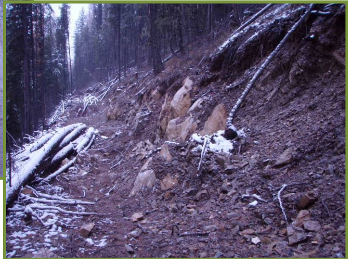
Photo 2 (below) 2007 pilot trail, no subsurface drainage was intercepted (November 6, 2008).
