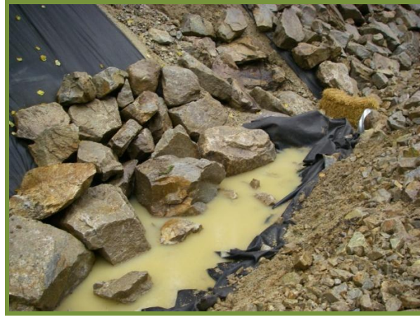
Suspended clay in standing water at station 192. Note geotechnical filter fabric.
