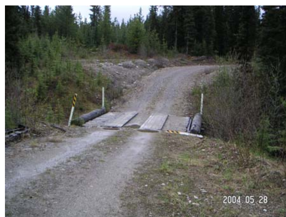
Figure 3 - Bridge K-1051 – not load rated, although MOF inspections note significant rot in stringers. One of the bridge delineators is knocked down.
