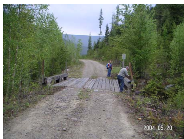
Figure 4 - Bridge N7-114 – no load rating sign or bridge delineators.
