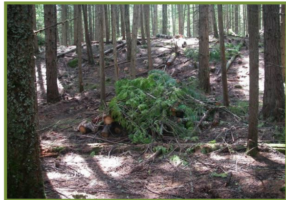
Treated stand at Kaslo. Deciduous and large Douglas fir were preserved. The conifer understory was removed. Thinning targeted clumps of regeneration under the canopy of larger trees. Trees were pruned to 2 m. This debris is waiting to be burned.
