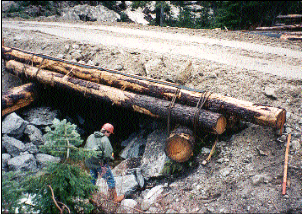
Bridge construction and maintenance are key areas of examination in Forest Practices Board audits.
