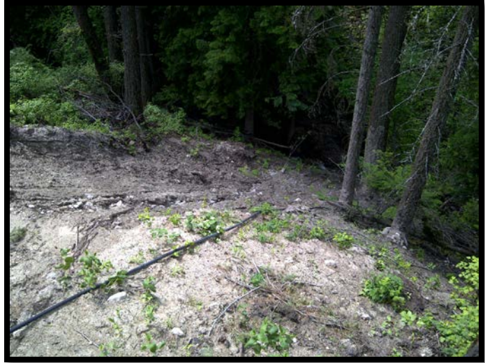
Photo 2. The slide extends into Gilpin Creek.
