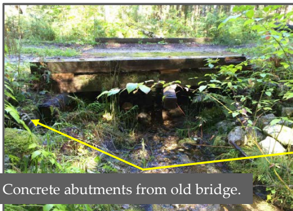
Figure 4. Old bridge with deteriorating wooden deck and stringers. The wood stringers rested on concrete abutments.
