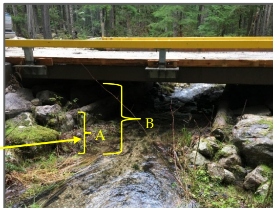
Figure 5. New bridge November 2016. (A) is the height of the old bridge and (B) is the height of the new bridge above Malakwa Creek.
