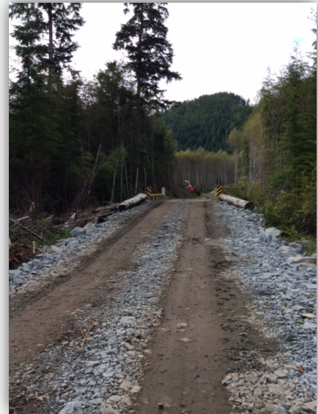
New road and bridge construction. The bridge is elevated to drain water away from the crossing.
